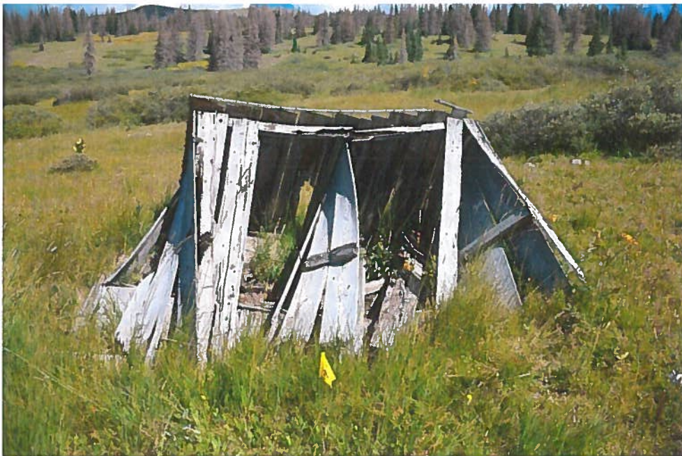
Figure 36, Building #26, Collapsed 2 hole/2 door Privy. Looking north.
