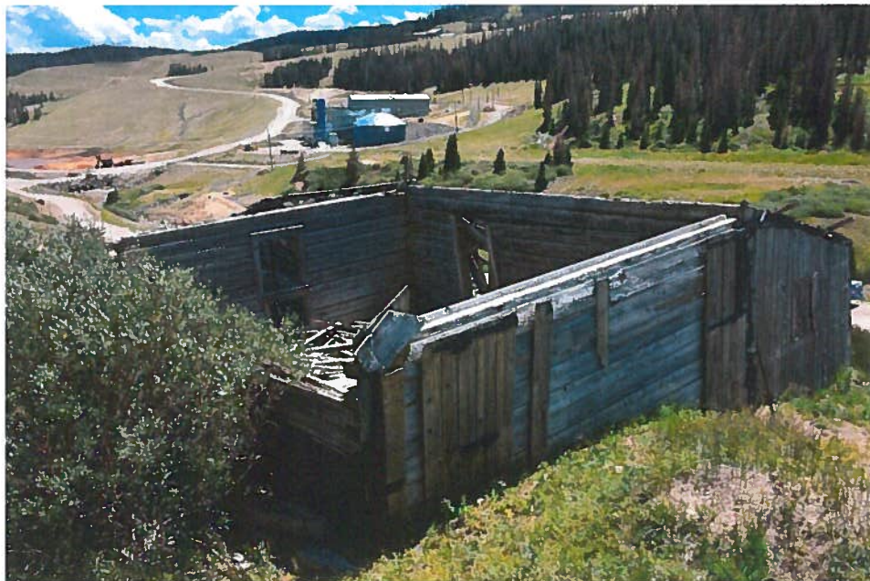
Figure 43, Building #33, Roofless building, of similar design as the others, 44' (NW/SE) x 40' (NE/SW). Sits 330 feet SE of main group, and Building #13, over looks main road. Looking SE, EPA Treatment Plant in background.
