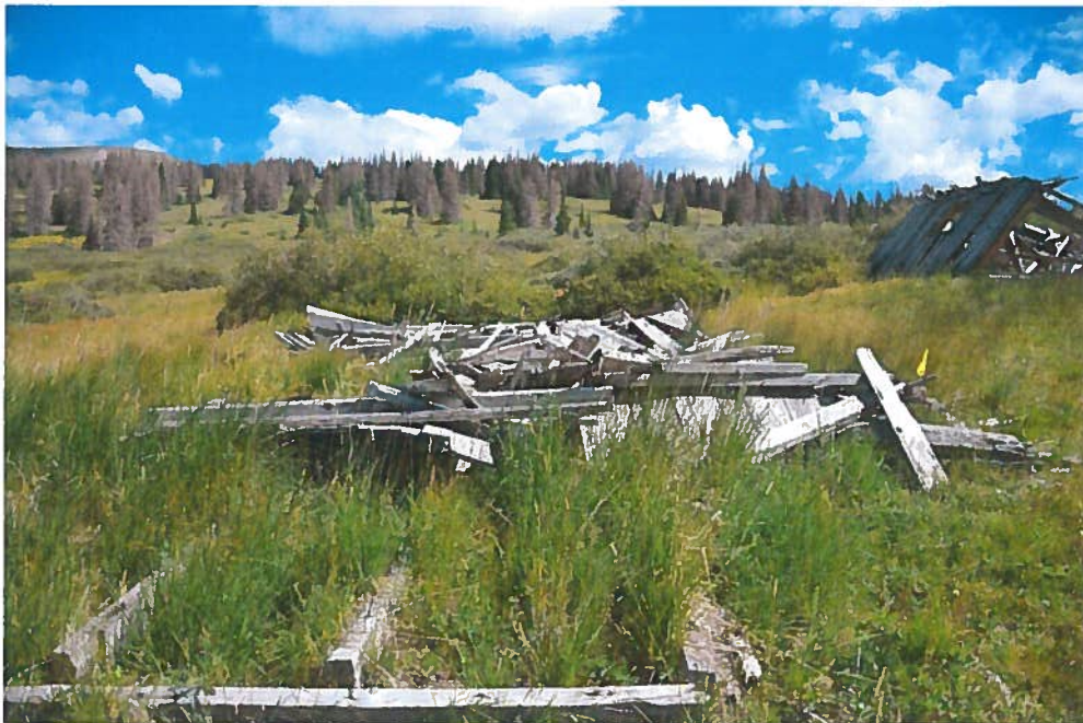
Figure 34, Building #24, collapsed residential structure. 19' x 14'. Possible lean-to addition on south side. Looking north.
