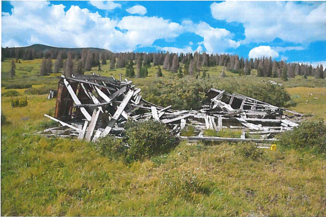
Figure 33, Building #23, collapsed residential structure, 29' E/W on south wall, 17' N/W on west wall, 24' N/S on east wall. Looking north.
