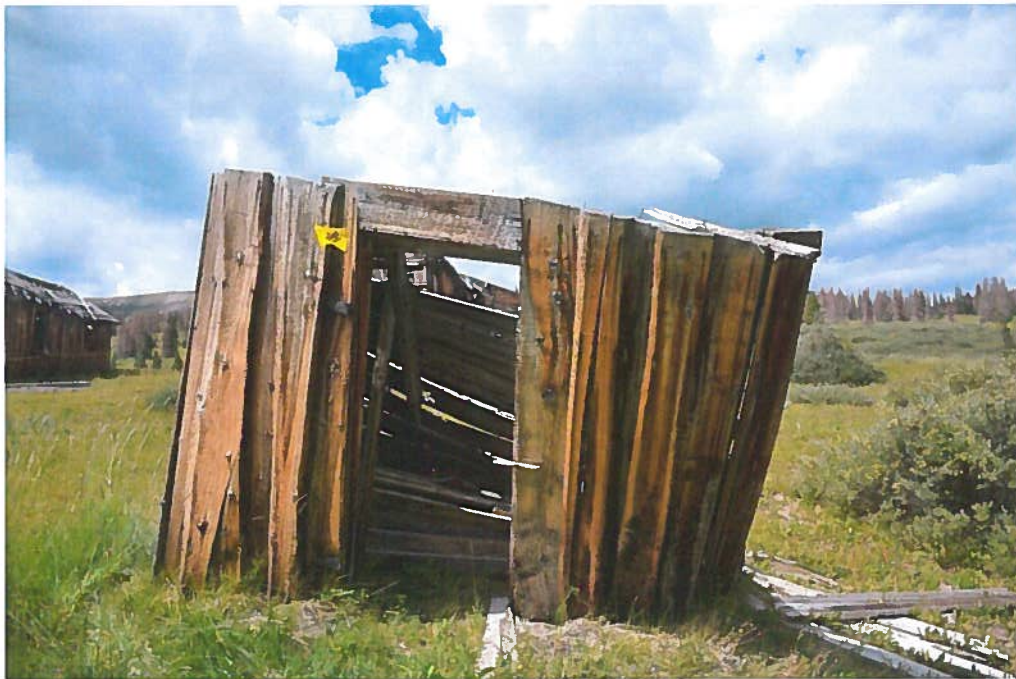
Figure 28, Building #18, Hydrant House, same dimensions as others, warped. Looking north.
