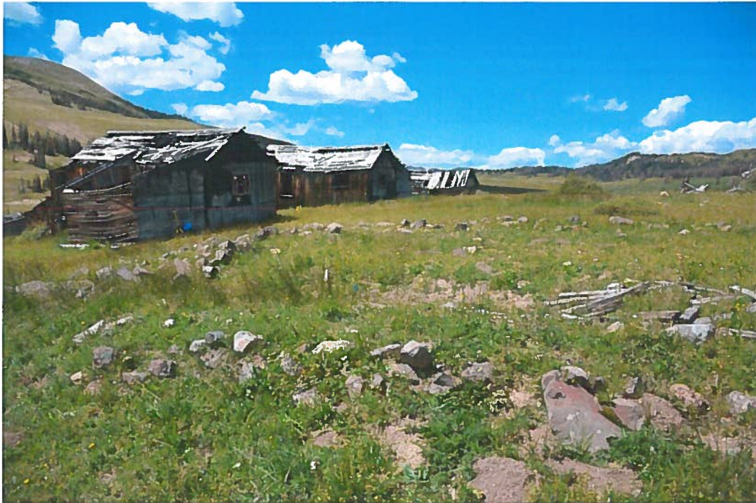
Figure 42, Structure #32, Rock lined depression, possible cellar. 38' x 32'. Rock foundation wall is about 6' ft. wide on the side and east side, slightly smaller on west side, and absent on north side. Parts are 5-6 ft. deep. Looking southwest.
