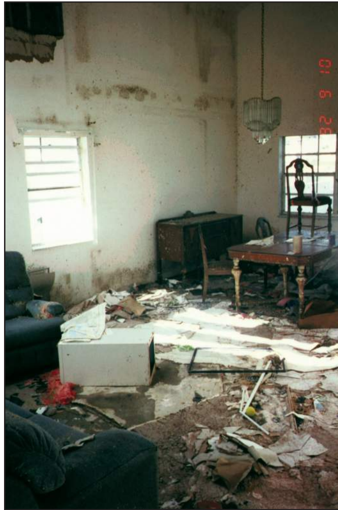
Figure 4 In low-lying areas, wind and rain damage to interior finishes and furnishings was exacerbated by flood waters.
