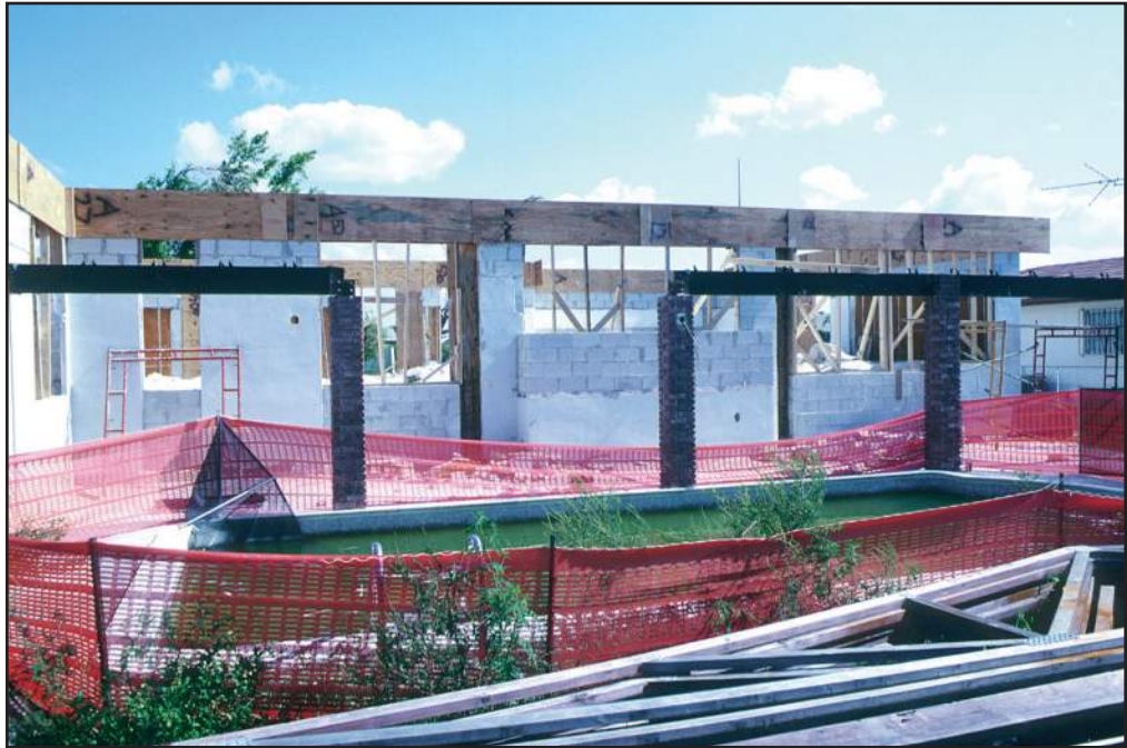
Figure 23 View from the back of the house. The walls have been extended upward with concrete blocks. The plywood visible at the tops of the walls is used to form cast-in-place concrete bond beams that will strengthen the extended walls. The roof trusses shown in the foreground were salvaged for reinstallation. The owner of this house decided to replace the original roof sheathing and shingles with new materials.
