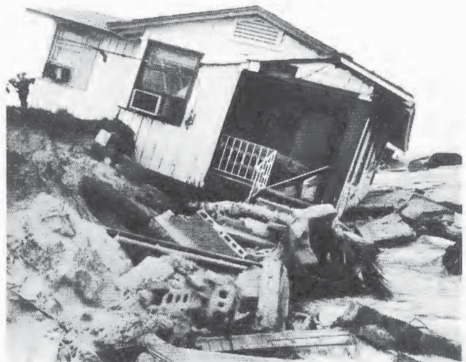
Figure 2.3. Erosion Caused This Foundation to Collapse.
